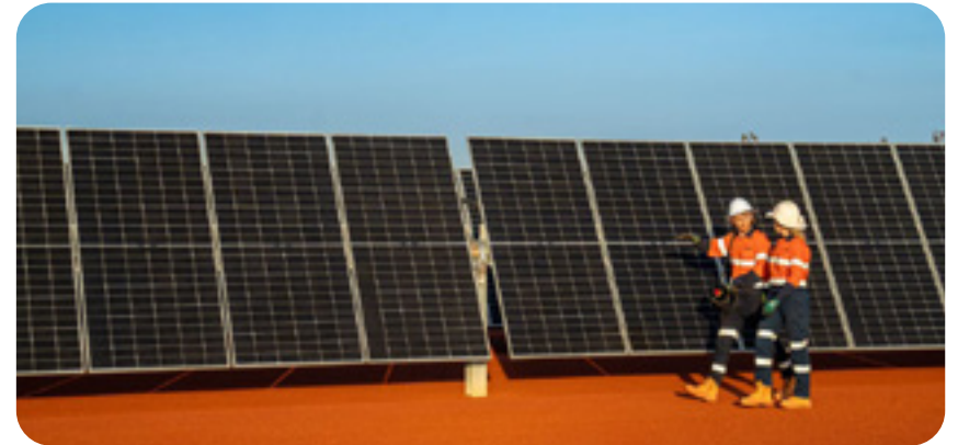
Rio Tinto Weipa renewable energy microgrid
